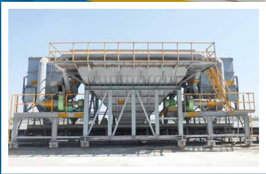
Ruby Cement: Fabrication, Erection & Commissioning of 04 Nos. Eco Hopper at Patanga, Chattogram.
